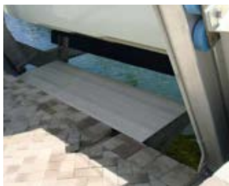
Elevator Boarding Platform
